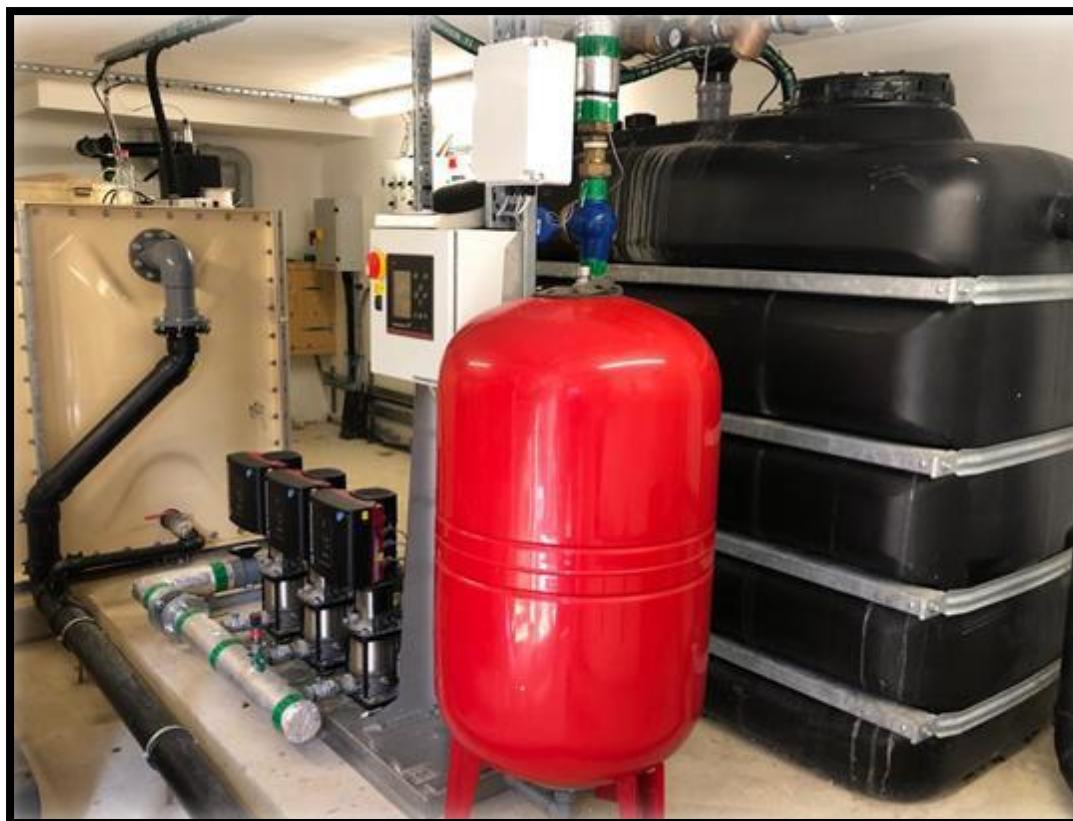
Image 3.3 Courtesy of Aquality – Clay Farm plant room
